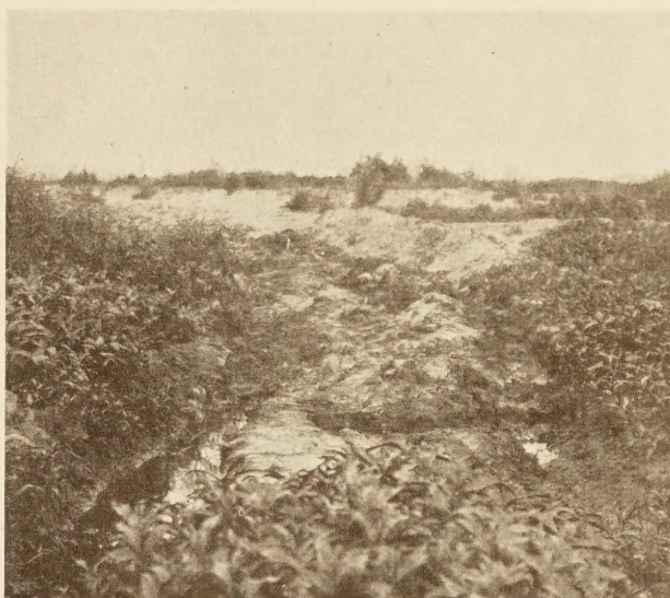
FIGURE 2.—WET AREA AT STATION 20+00. POWER SHOVEL WAS STUCK AT THIS POINT
